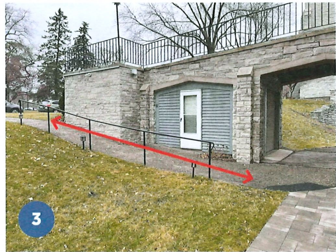
INACCESSIBLE ENTRY PATH (APPROX 1:6 SLOPE)
