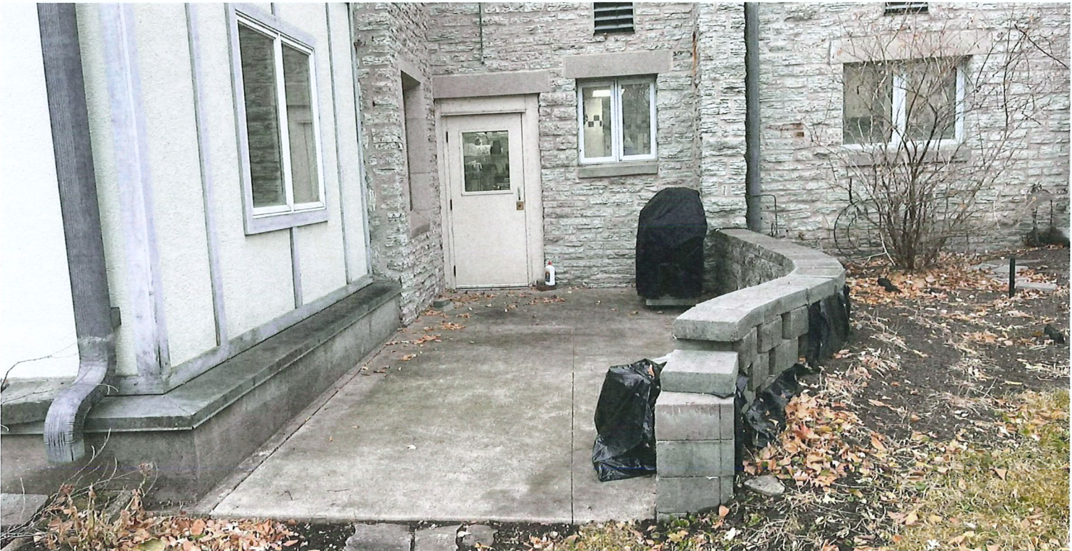
KITCHEN DOOR WITH FLOODING ISSUES TO BE REMOVED
