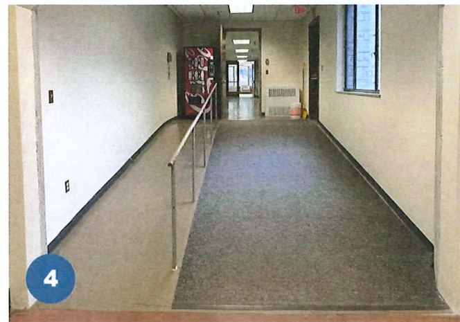
LINK RAMP SLOPE 1:8 NON ADA COMPLIANT
