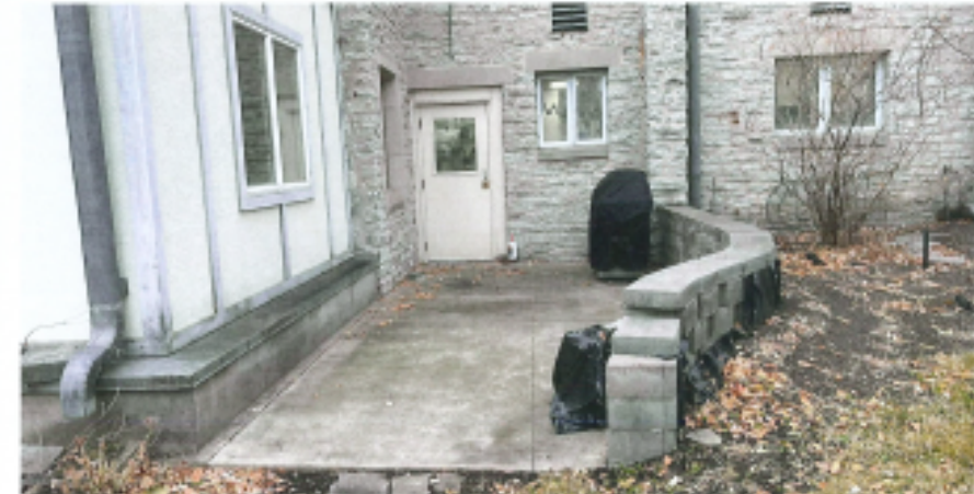
KITCHEN DOOR WITH FLOODING ISSUES TO BE REMOVED
